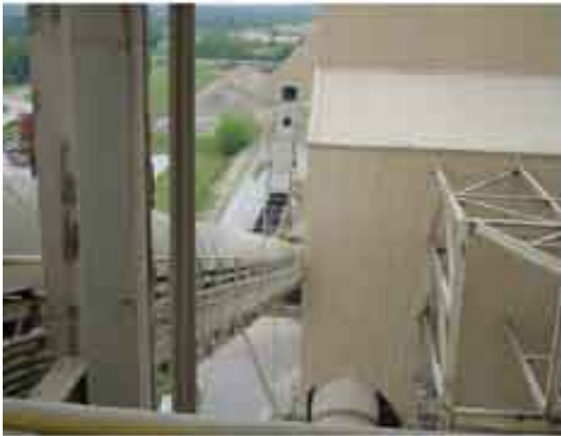
Conveyors to Kiln
