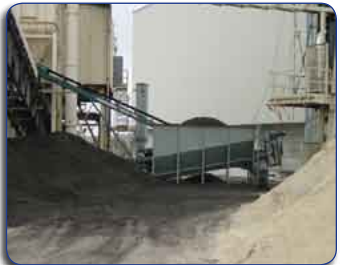
Metering system to introduce TDF into wood mixture before processing Photo courtesy of Terry Gray, TAG
